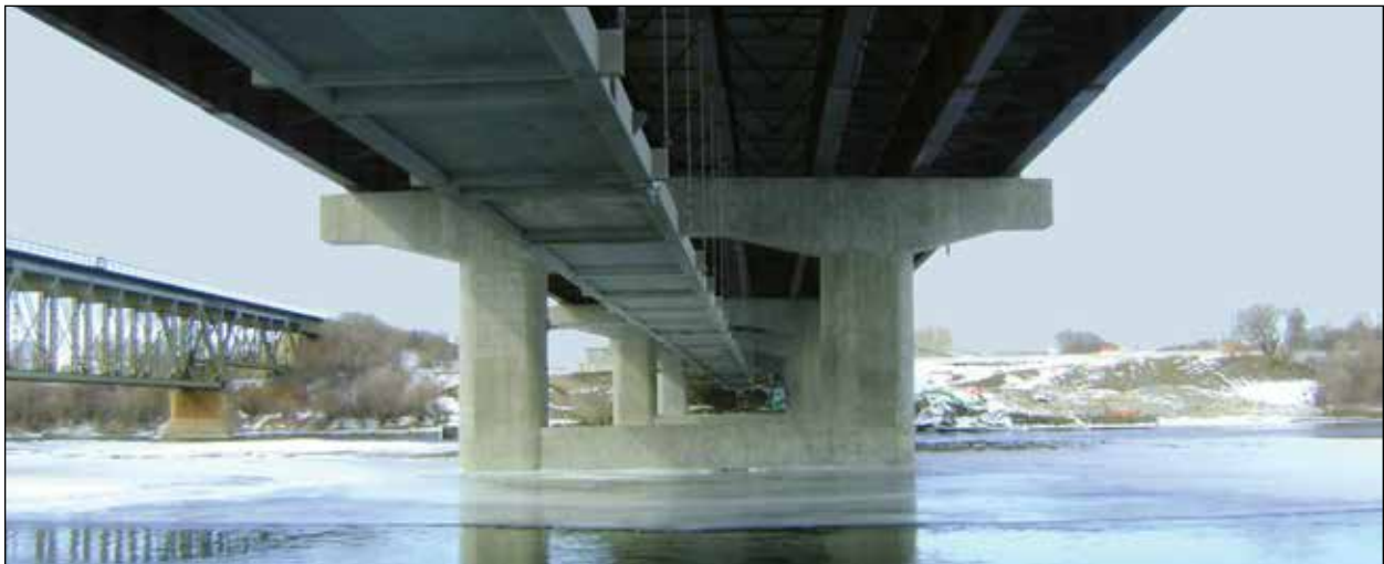
Circle Drive over South Saskatchewan River - Saskatoon, SK, CAN ChromX steel used to construct six-lane bridge deck and columns. Constructed 2012
