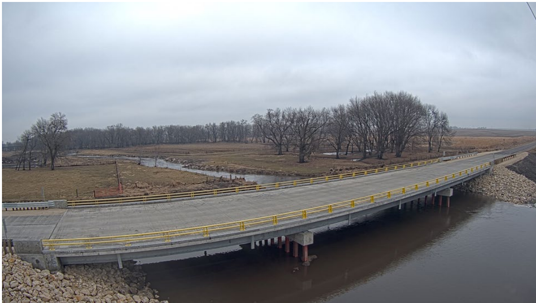
Figure 33 Buffalo Creek Bridge in Independence, Iowa GalvaBar was used in the Abutments and Parapets of this Bridge
