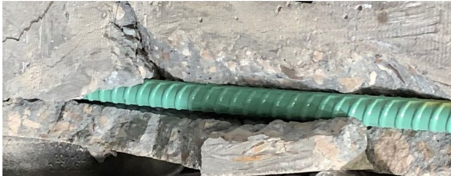
Figure 29 Lack of Bond Between Epoxy-Coated Bars and Concrete Under Static Loading
